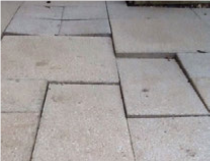
Poor bedding layer
