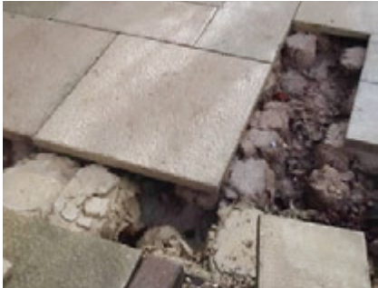
Spot bedding giving poor support
